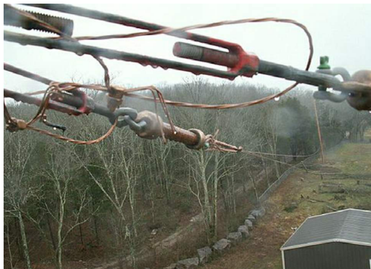
A close-up view of the turnbuckles and support system for one of WTWW's massive rhombic arrays. (Courtesy: John Hettish – Middle Tennessee Two-Way, Inc.)
