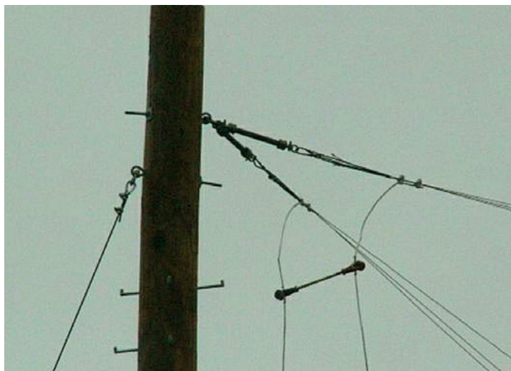
A telephoto view of how the twin lead feed line connects to the feed point of one of WTWW's huge rhombic antennas. (Courtesy: John Hettish – Middle Tennessee Two-Way, Inc.)
