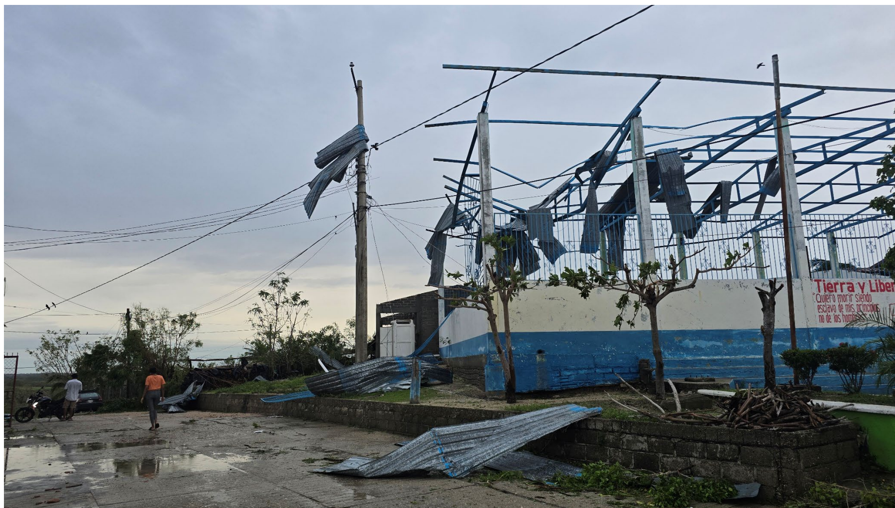
Figure 11. Entire metal roof destroyed from recreational space building in San Jose Estancia Grande, Oaxaca, Mexico, following the landfall of Hurricane Erick. Image courtesy of Josh Morgerman, iCyclone.
