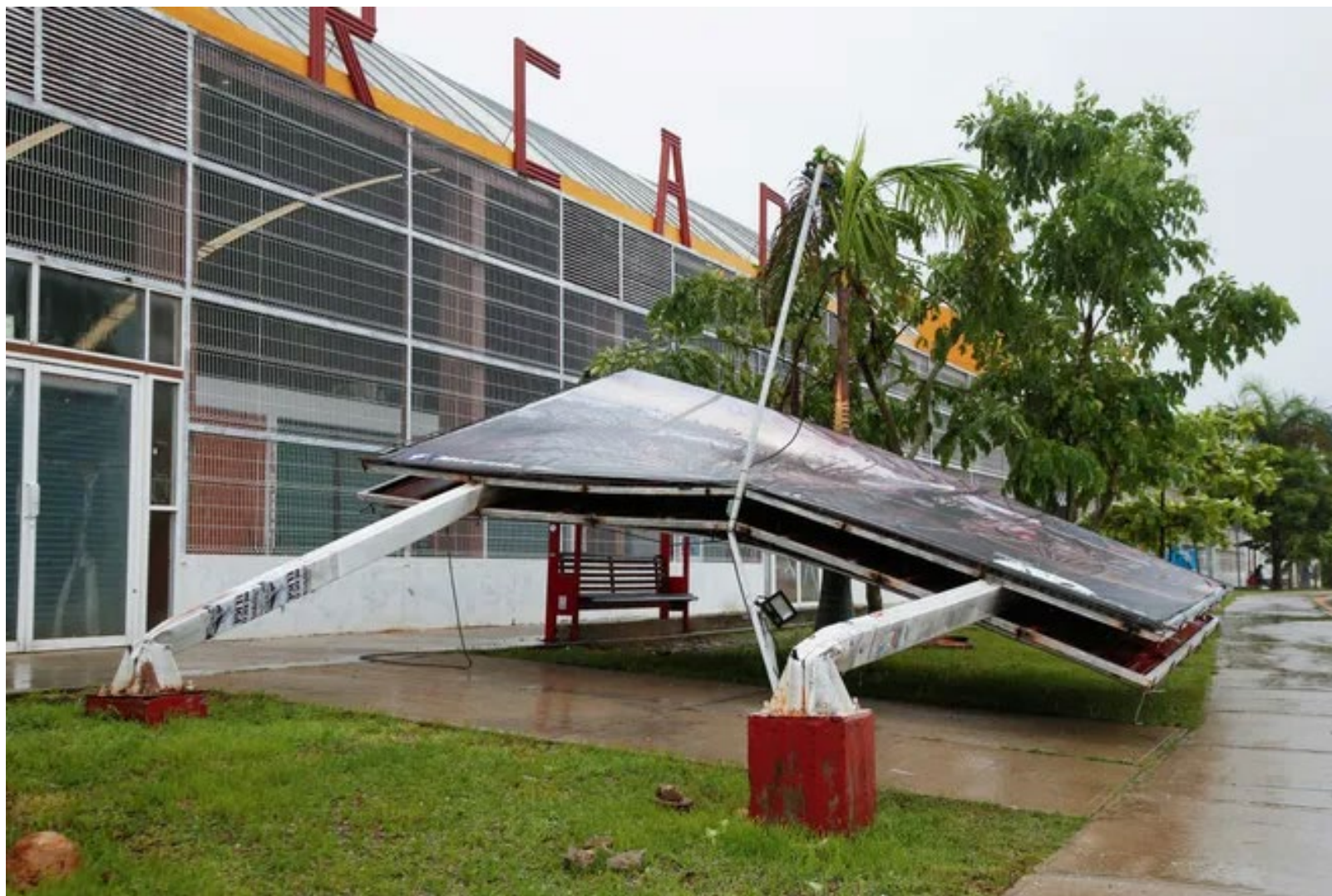
Figure 14. A billboard knocked down in Puerto Escondido, Mexico following the landfall of Hurricane Erick. Image courtesy of Jorge Luis Plata, Reuters.
