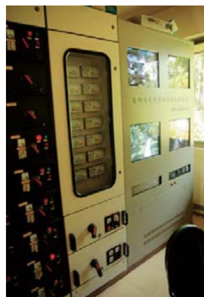
Fig. 6a-2 The monitoring system for the dredging and improving project of Changqiao Stream, photographed in 2008
