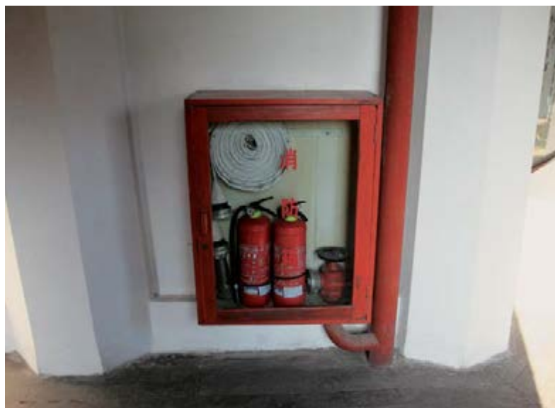
Fig. 4a-12 Fire hydrant inside Liuhe Pagoda, photographed in 2008
