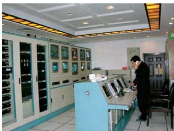
Fig. 6a-3 Monitoring Room for the safety of Leifeng Pagoda, photographed in 2002
